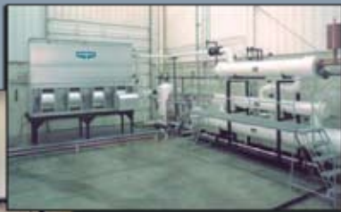
Condenser Test Chamber
